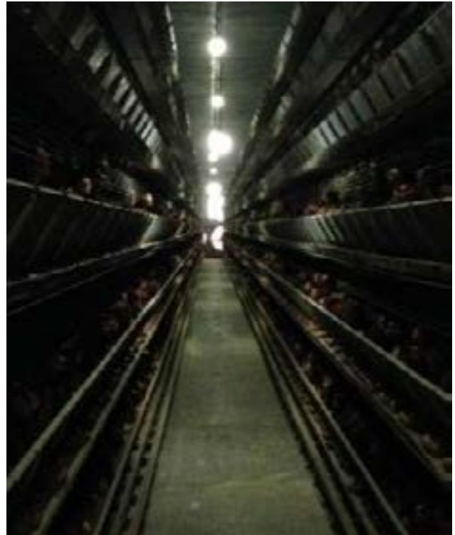
Figure 18. The LED lights installed in this house are too directional, too far apart and not bright enough. The combination of these factors leads to the obvious shadows on the floor and poor light uniformity along the cages.
