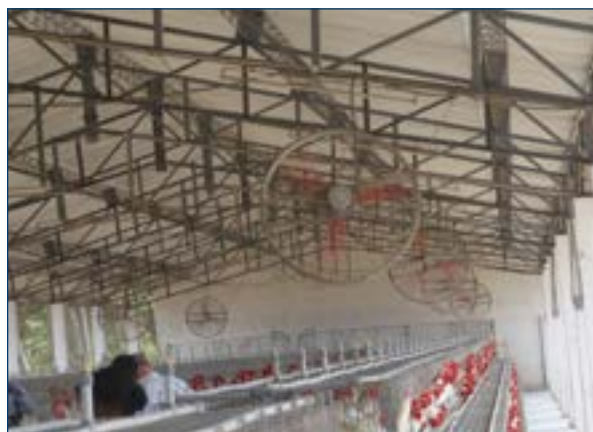
Figure 4. Stir fans and foggers increase air velocity within the house and create a cooling effect.
