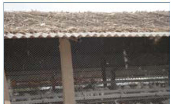
Figure 8. Use of thatching material (paddy straw, corn stalks, sugarcane tops) to reduce solar heating of the roof.
